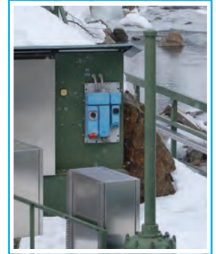
Hydroelectric power plant
