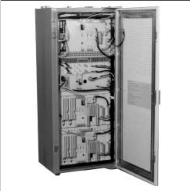
Base station of cellular network
