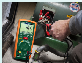
Insulation test on pump motor
